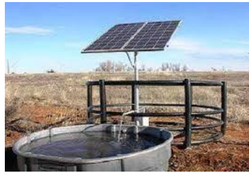
Figure 12 Application for Water pumping
